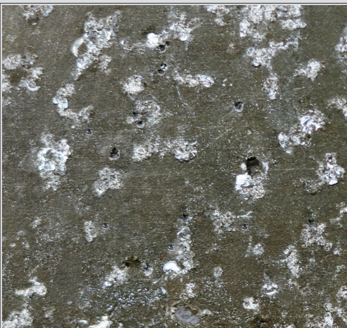
Details of surface corrosion
